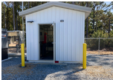
Booster Pump Station
