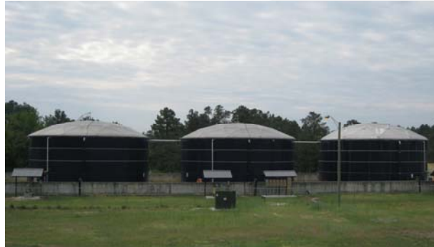
Storage Tank Farm
