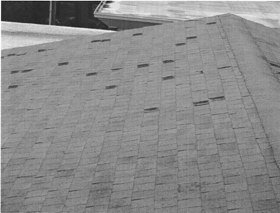
Photo 3 shows loss of shingle tabs (typical on both schools)
