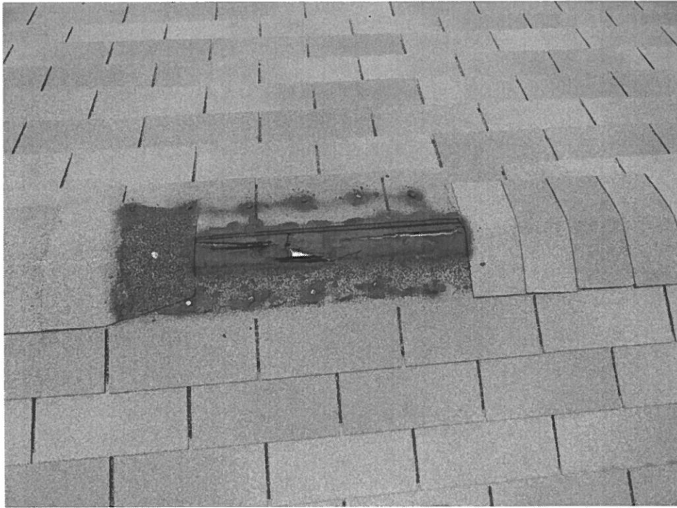
Additional repairs are needed on Building 600 on the Butler Campus, Photos 9 and 10
