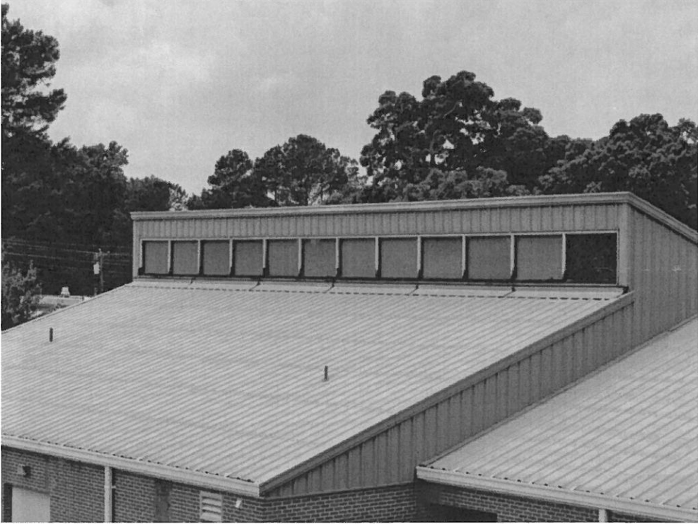
Photo 8 Leaking windows on adjacent roof
