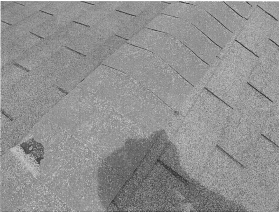
Photo 4 shows widespread granule loss at L. C. Kerr leading to accelerated shingle UV degradation
