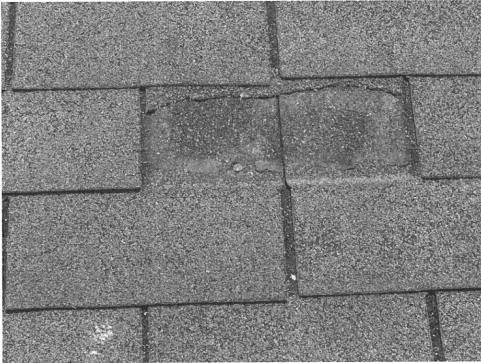
Photo 5 improper nailing of shingles (typical on both schools)
